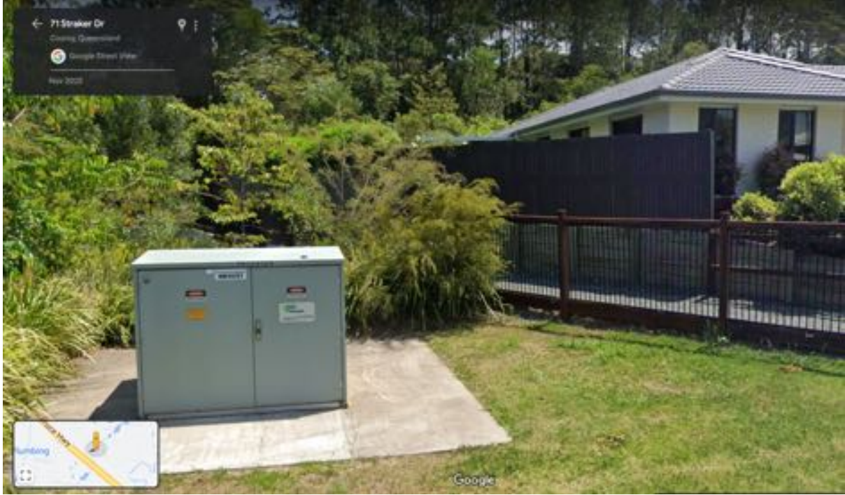
Found a Padmount Transformer
