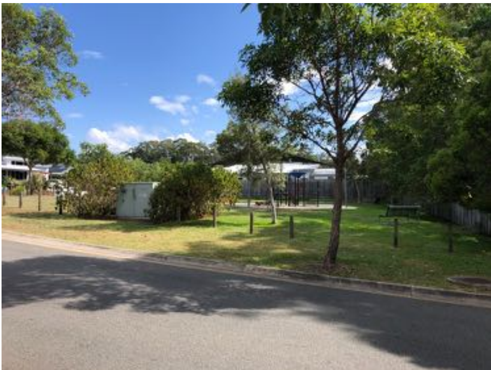
image of location – view of padmount
