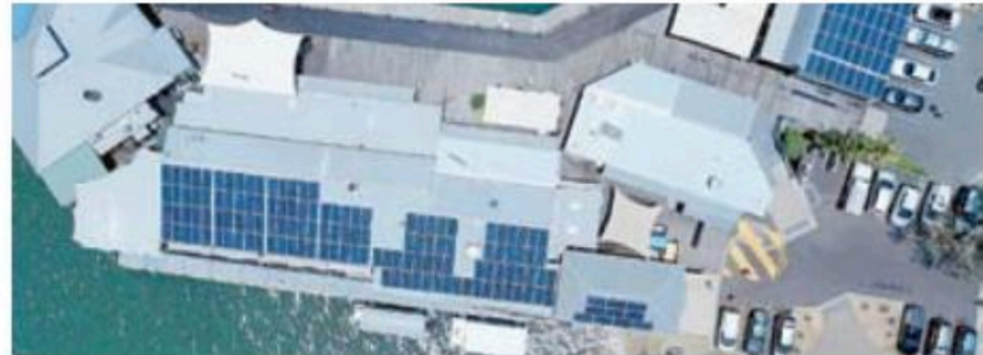
Solar panels on Marina roof.
