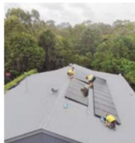
The Colefax installation.
